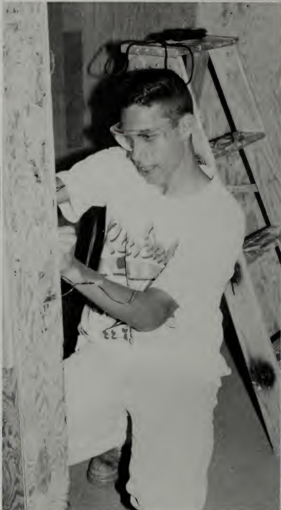
Tony Colarusso wires a panel box in the electrical shop. This wiring job was a required job necessary to pass the course.
